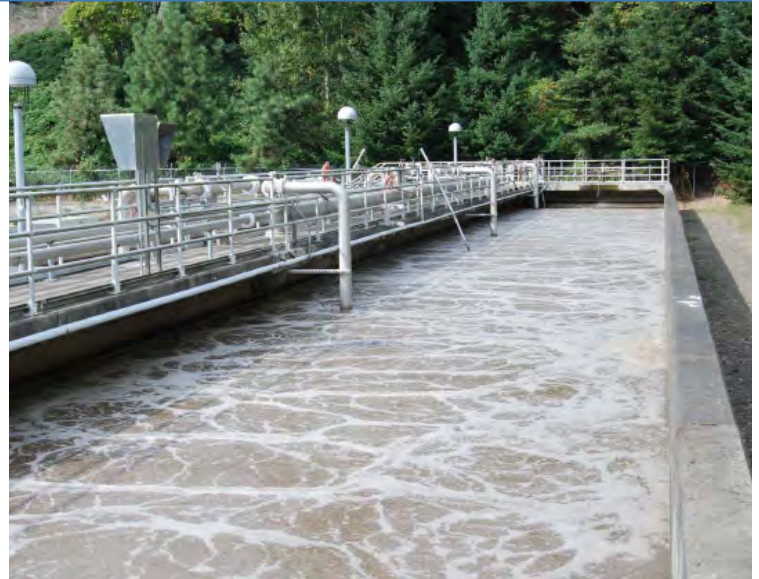
Wastewater is treated to rigorous state and federal standards, before being discharged to the Willamette River.
