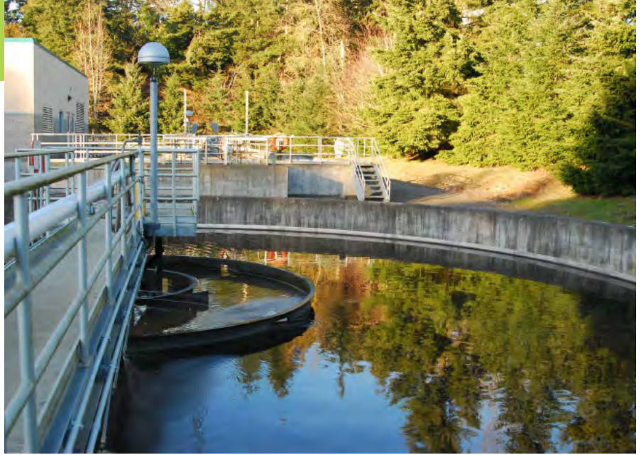
Built in 1971, Wilsonville's wastewater treatment plant is being upgraded to meet community needs and environmental regulations.
